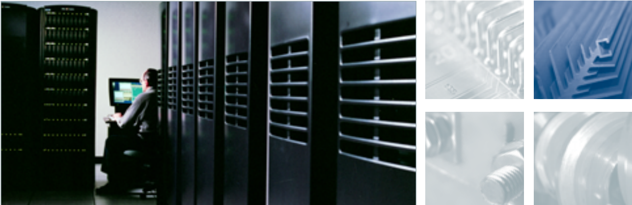
Computer server room
